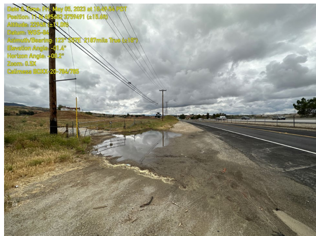
Ponding water, same area as previous photo, facing east-southeast (05.05.2023).
