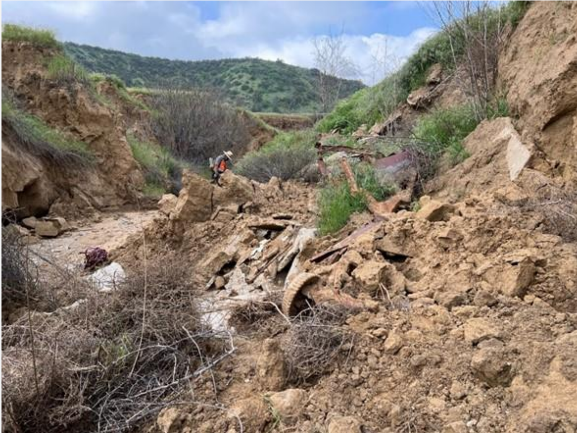
Figure 10. Overview of MV-S-003, refuse in a drainage, facing south.
