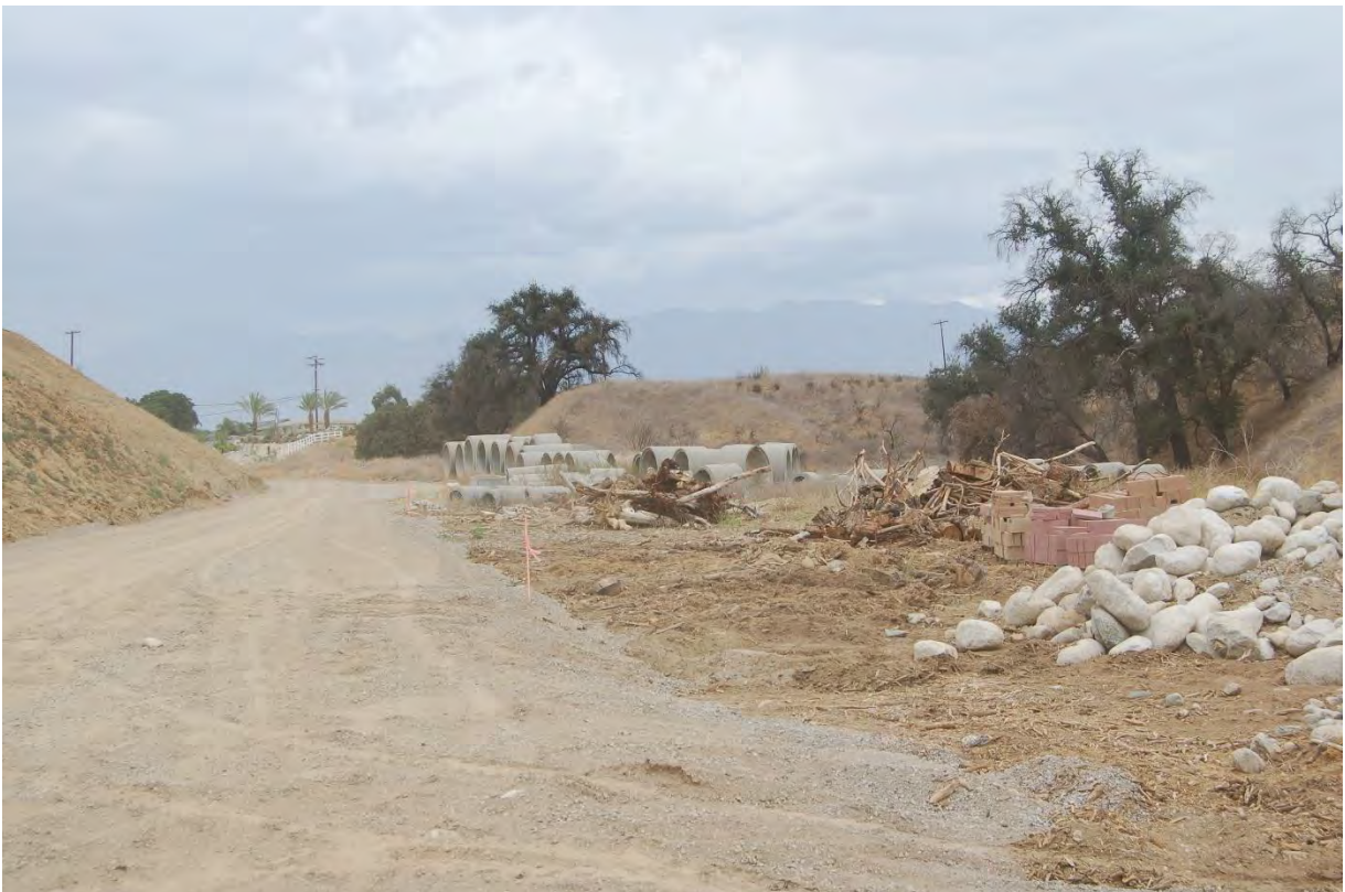
Photo # 8 – Stockpiled concrete pipe, brick, cobbles and general debris along dirt road below trailer park.
