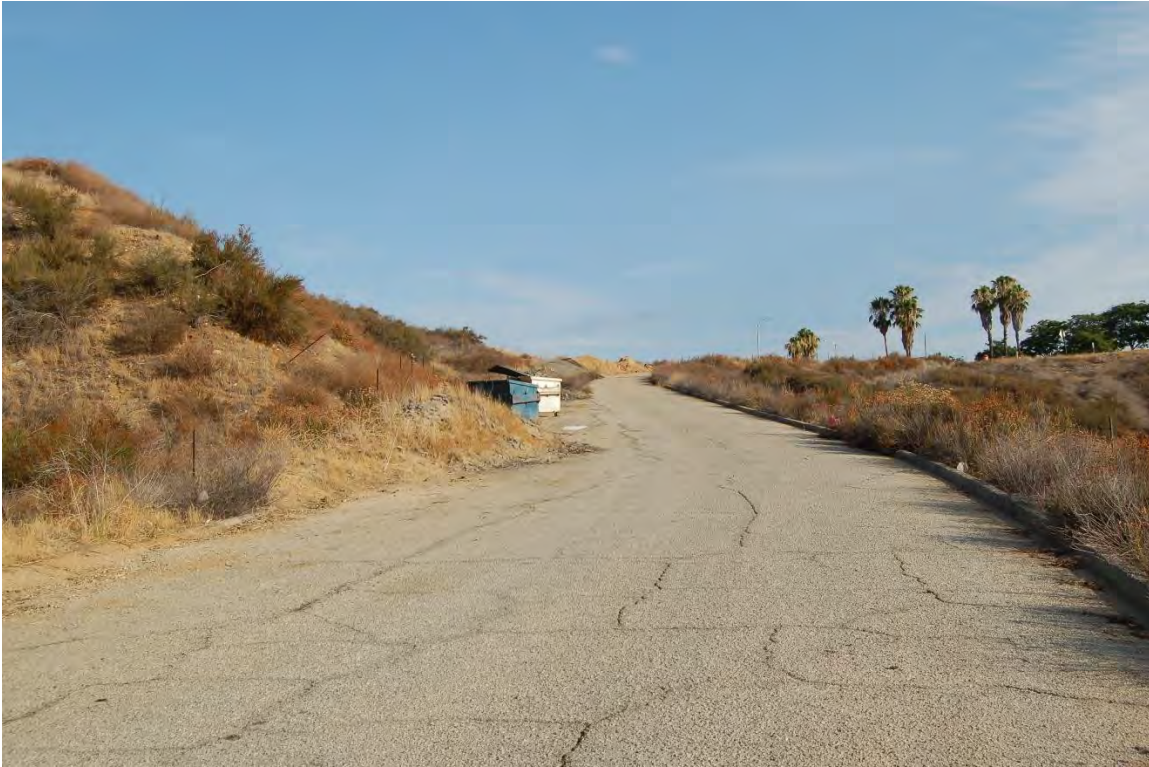
Photo # 3 – north view of upper portion of Shady Brook Road. Note stockpiled asphalt and soil in background behind trash bins.
