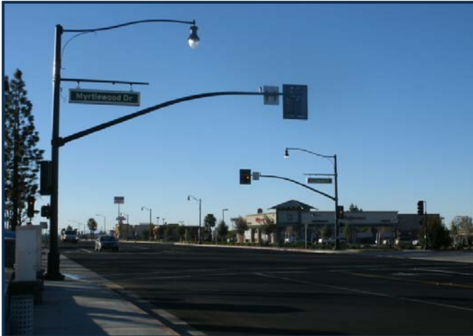
The signal at Myrtlewood Drive and Calimesa Boulevard is part of the City's overall system of traffic controls.
