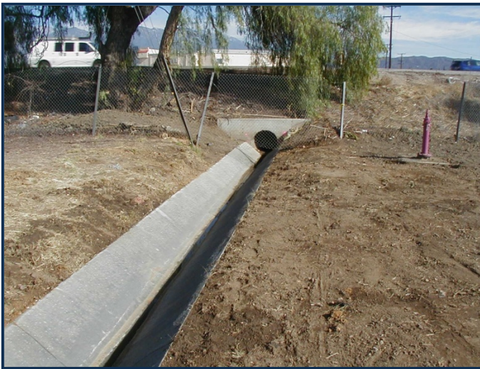
The storm drainage system in Calimesa includes large creeks and channels, and small facilities like this one.
